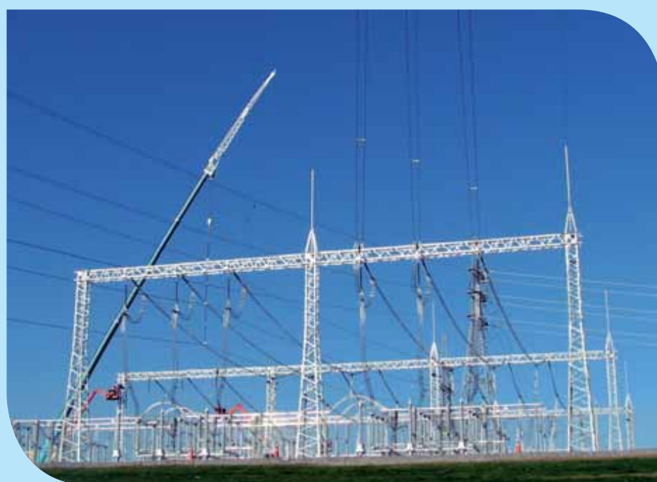
With the help of a crane Electrix pioneered the lifting of live transmission lines. This allowed the construction of a new substation below the lines while maintaining the supply of power.
