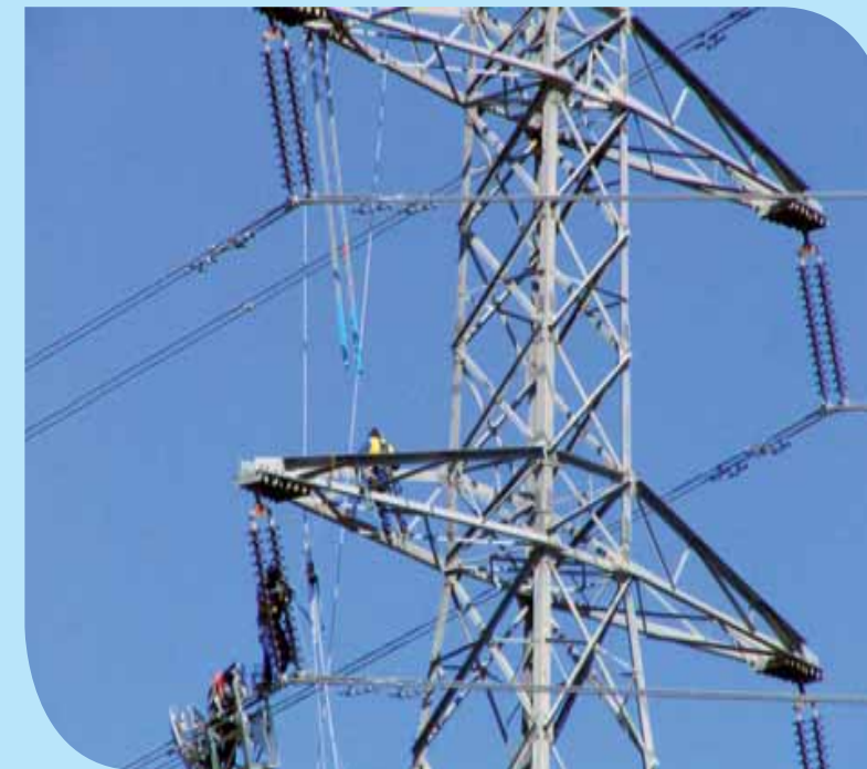
Electrix mobilised resources at short notice to replace insulators on a section between the vital Huntly-Otahuhu line.
