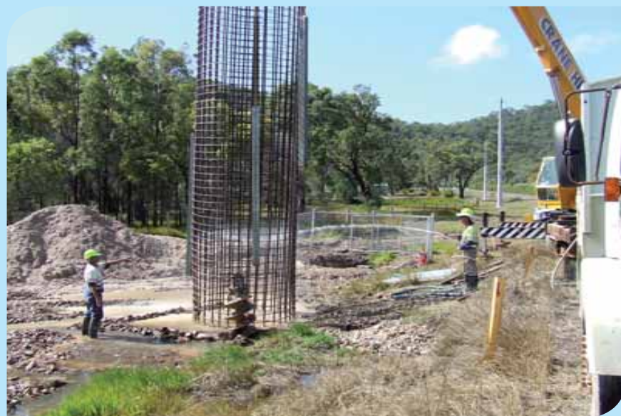
On Queensland's Discovery Coast Electrix overcame a number of obstacles when they designed and built a new 47km transmission line.
