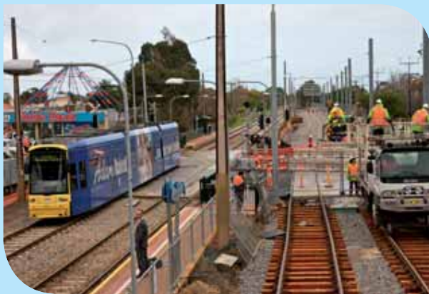
The track realignment and new overpass for the Glenelg tram is an important local infrastructure project and a successful debut for Electrix' in the rail sector.
