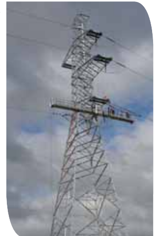
Electrix' modified strain working platform improves safety and efficiency. Linesmen can now carry out 'dead-ending' from the safety of a suspended platform that is securely anchored to the tower and ground.
