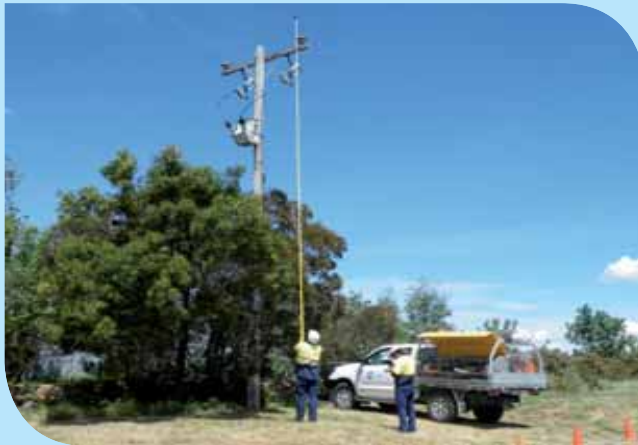
Electrix is adding value through innovation as part of a substantial 3-year maintenance contract with two one-year extensions for Powercor and CitiPower.
